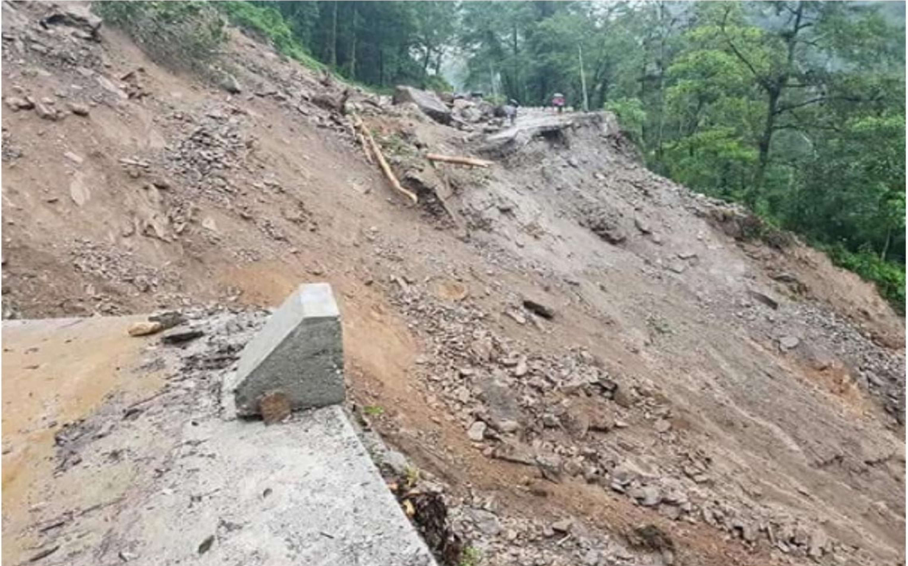
Landslide in North Sikkim disrupts road connectivity. Photo: Northeast Now Representative image
