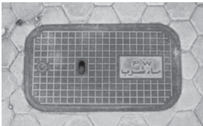
Potable water valve access box on sidewalk on Embassy Row in Riyadh, Saudi Arabia. Photo courtesy of Bahman Sheikh
