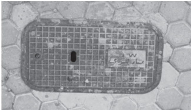
Reclaimed water valve access box on sidewalk on Embassy Row in Riyadh, Saudi Arabia. Photo courtesy of Bahman Sheikh
